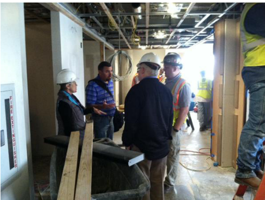
Dr. Richard Brettell meets with construction team at the Edith O'Donnell Institute's new UTD headquarters on February 20, 2015.
