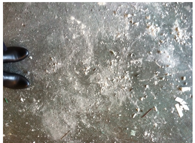
Site visit to the Edith O'Donnell Institute's UTD headquarters under construction on February 13, 2015.
